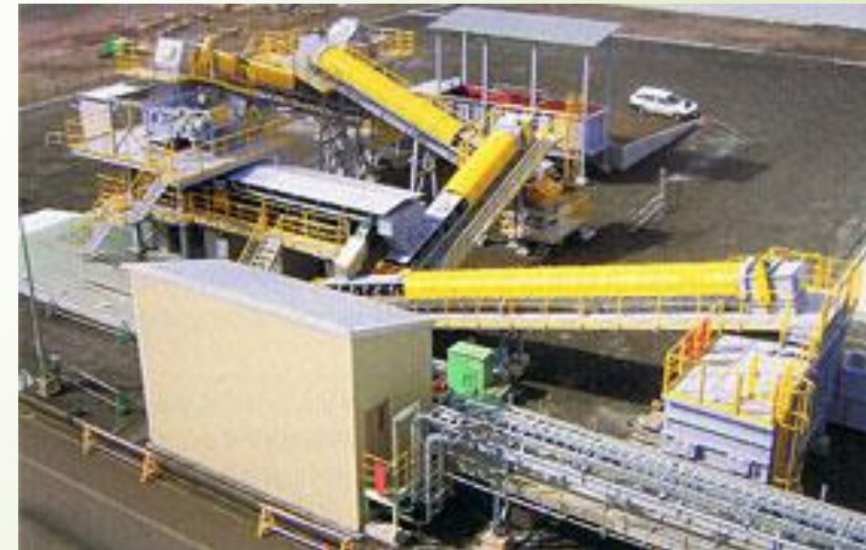
Waste Tires Shredding Facilities
