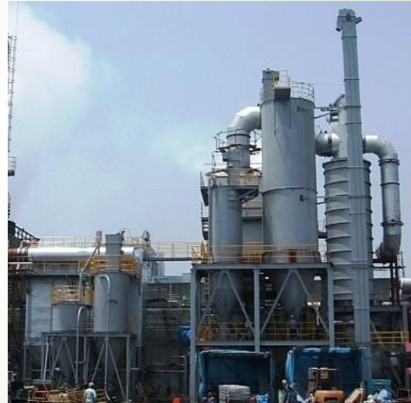
Exhaust gas treatment equipment for paper mills
