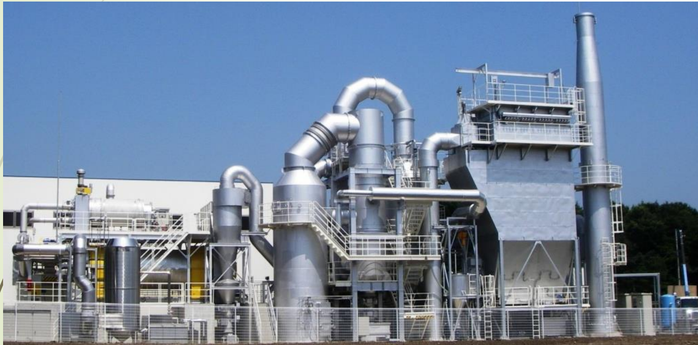
Sludge Drying Facility
